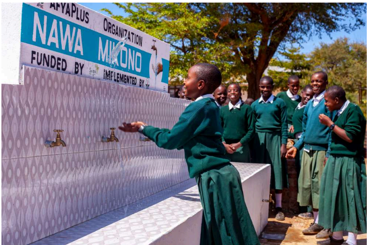
A student at Irole Secondary School using the newly installed handwashing station built by Afyaplus, promoting better hygiene in their school.
