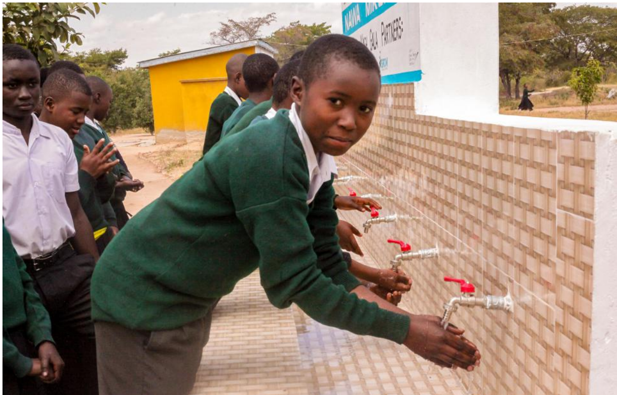
Fig 6: Hand washing station constructed at Kalenga Secondary School in Iringa Municipal it's in operation.
